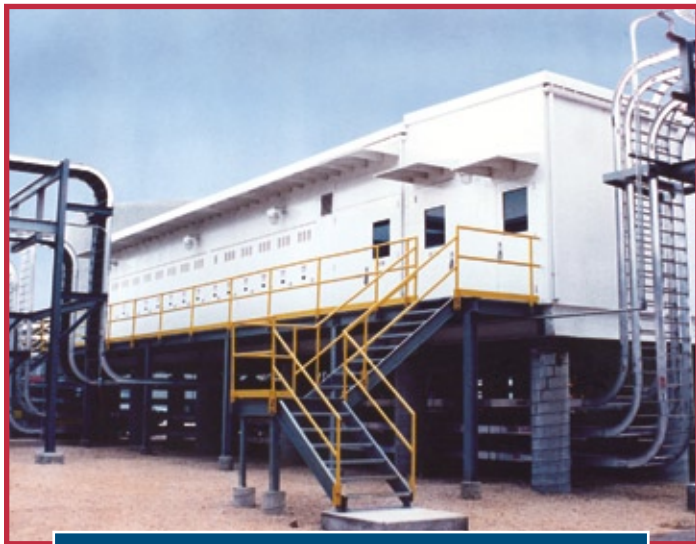
PCR installed on concrete piers at a gulf coast petrochemical complex.
